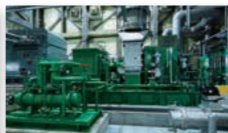
Steam Turbine Generator
